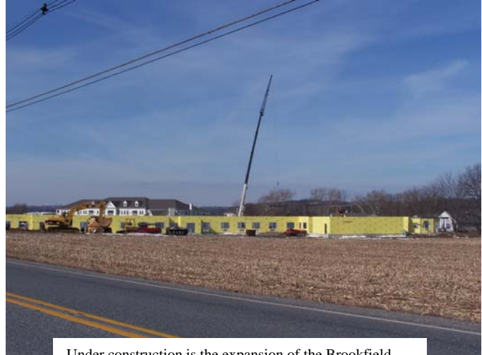
Under construction is the expansion of the Brookfield complex on Rt 519 in White Township
