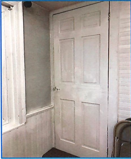
Soot coating on all interior surfaces: ceilings, walls, flooring and furniture
