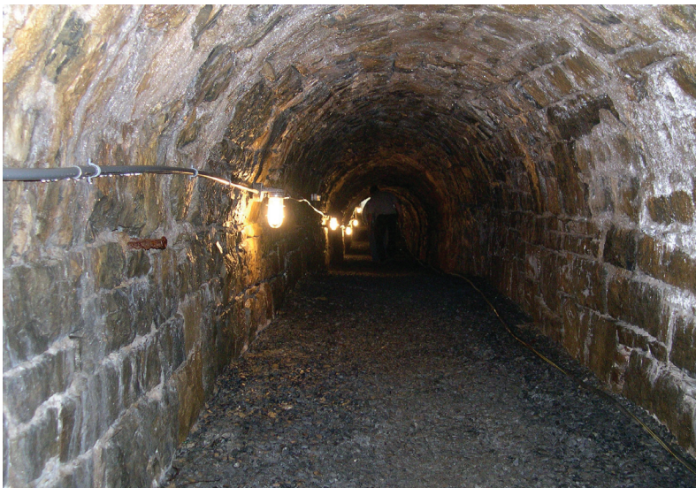
Looking up the tail race towards the Scotch turbine at Plane 9 West
