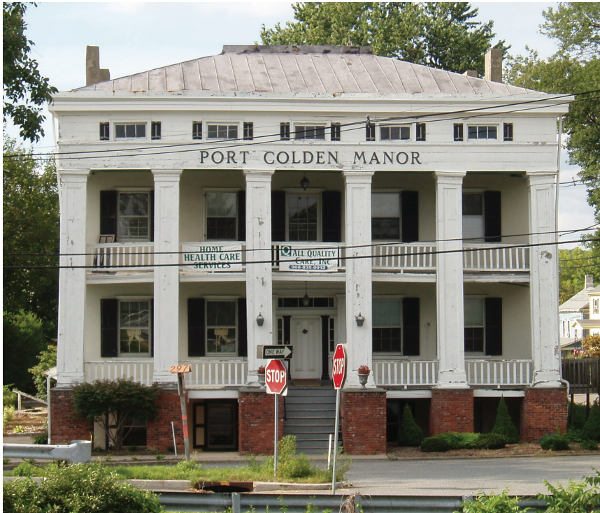
Port Colden Manor is a historic canal related structure in need of significant repair.
