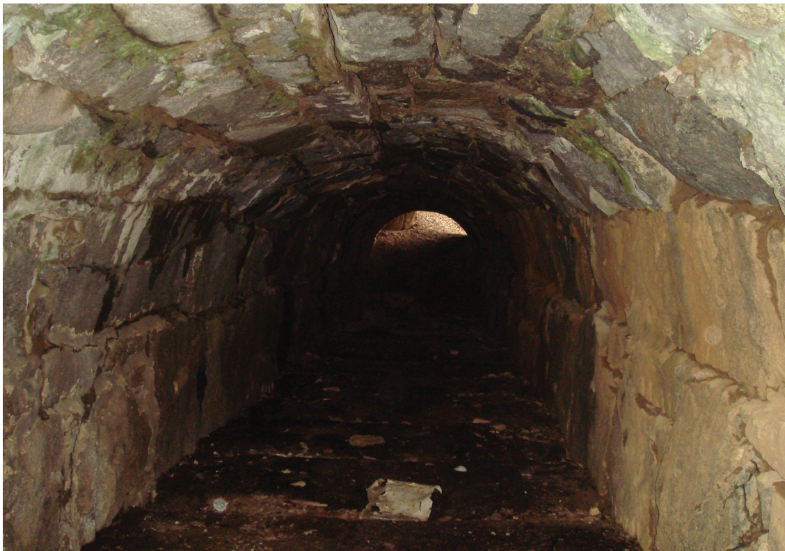
Looking down the tailrace at Plane 5W, also known as the Brickyard
